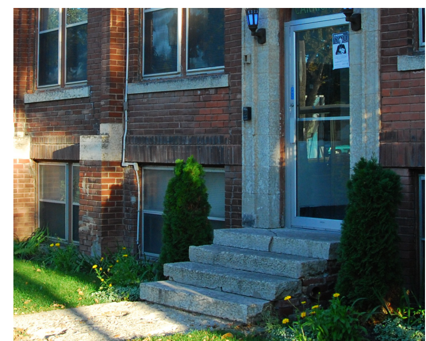
Building on Corydon with no wheelchair access
