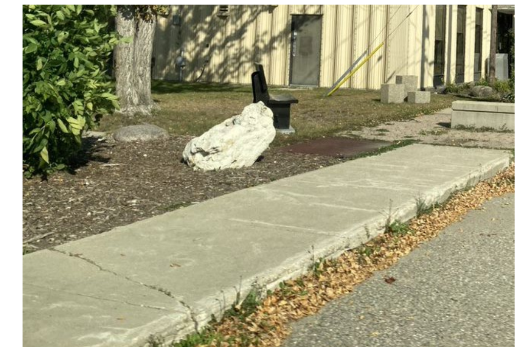
Fig. 34. Cracked sidewalk Photograph by Rudolph Nsoh
