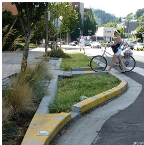
Figure: 24. Left: Stormwater curb bump-out (Hoboken)
